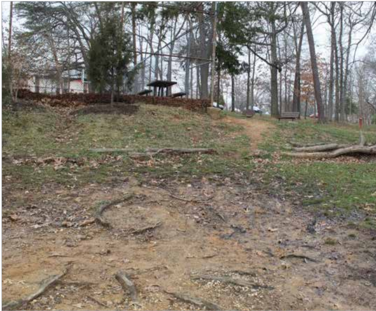
Erosion below the multipurpose courts
