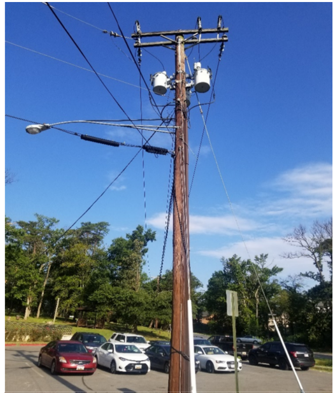
Onsite Power Pole
